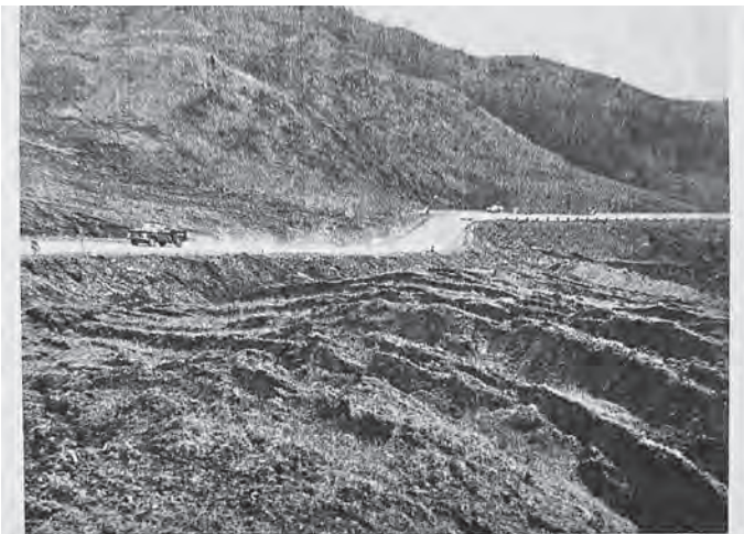
This doesn't look like the site of a million dollar slide at Hooskanaden Creek near Pistol River at the southern coast, now that a gravel road has been opened. But notice the deep cracks in the earth . . . they extend for half a mile toward the beach. The entire hillside slid toward the coast during the December rainstorms, destroying the road's alignment. This temporary road was built through the slide. Plans for finishing the road are underway. An
